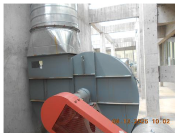
Waste gas facility.JPG
